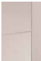
Particolare fresatura Close-up of machined groove
